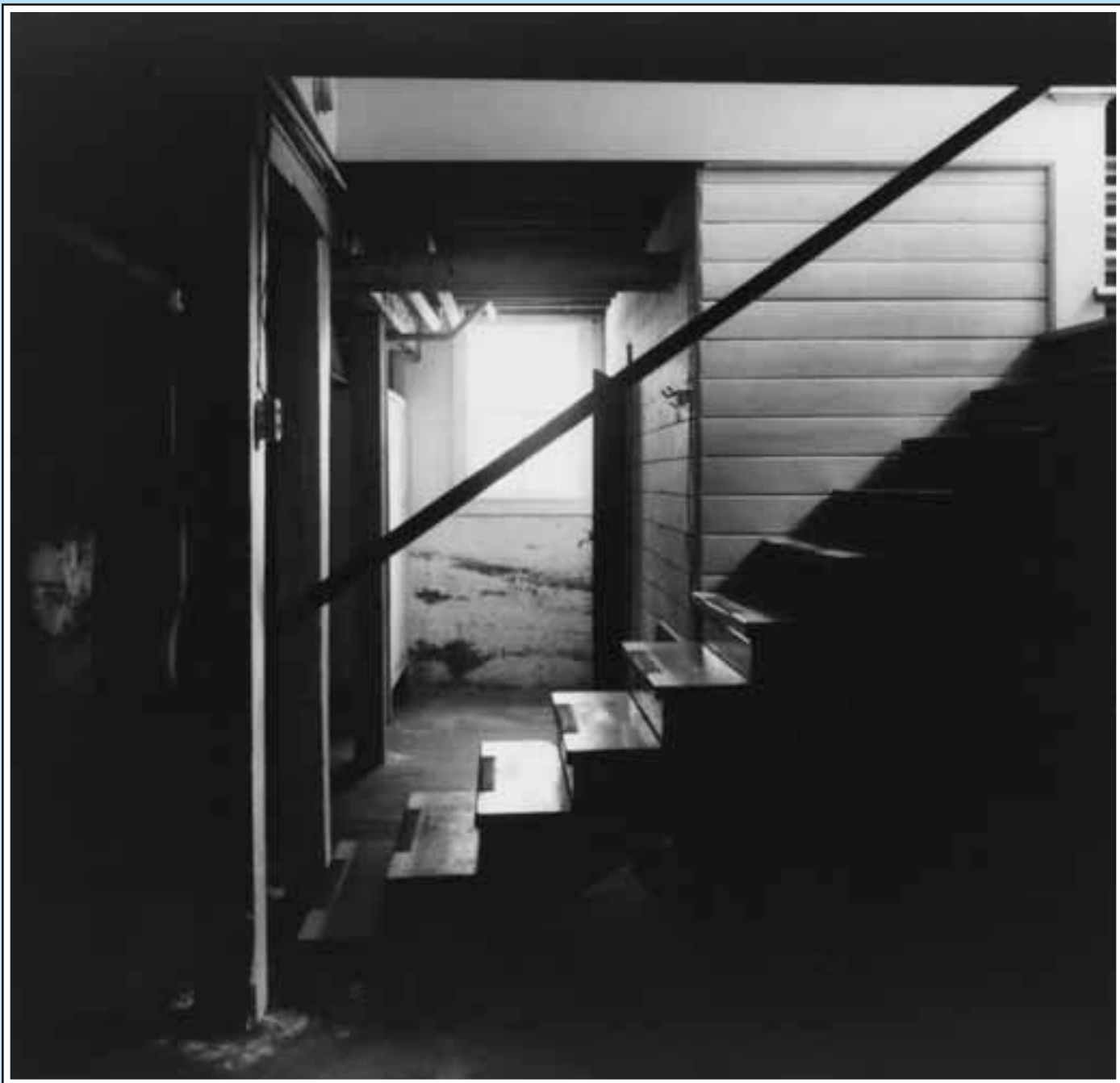
Parsonage Basement, Congregational Church of Faribault, 218 3rd Avenue Northwest, Faribault, Minnesota, February 1995
