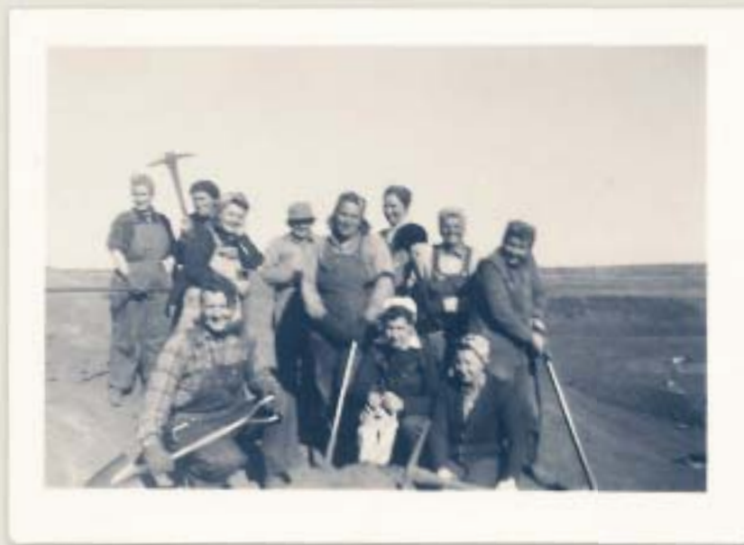
Track gang workers and "scrammers," who raked smaller rocks into piles that could be picked up by a loader
